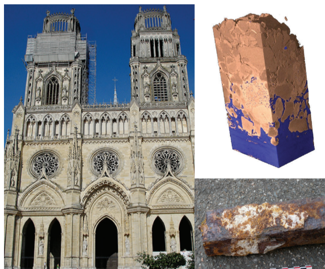
18 th century corroded metallic rebards from the Cathedral of Orléans (France) and 3D visualization of the corrosion interface (blue: metal, orange: binder). Their investigation may help to better understand long-term corrosion processes and compare corrosion product patterns in the case of atmospheric corrosion and corrosion in binders. (Image credit: LAPA)
